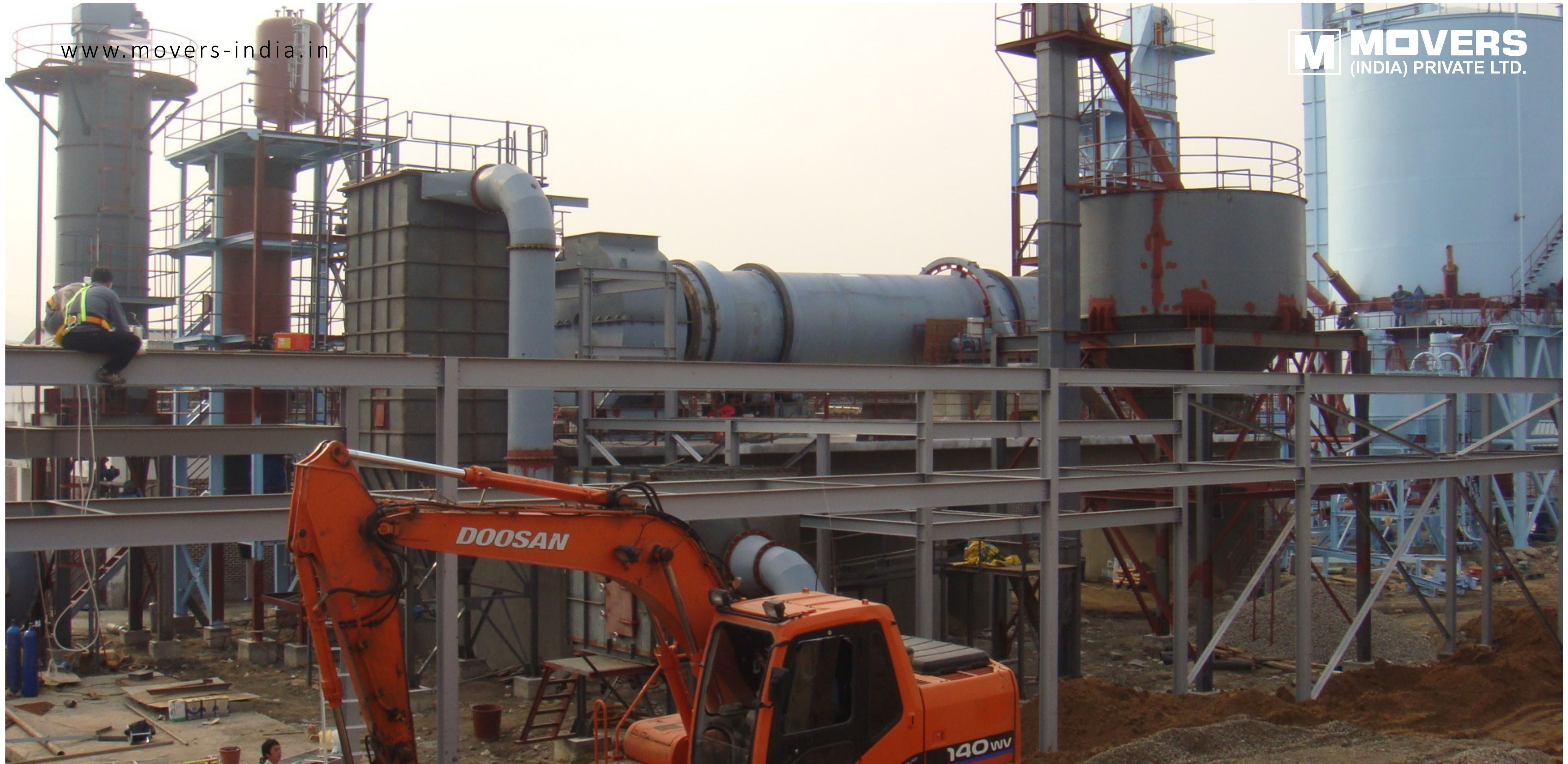
Photographs of W2E Plant
